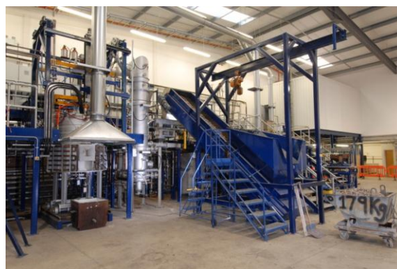
Gasification pilot plant
