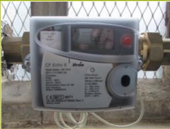
3. The probes on the meter have not been connected and so there is a zero meter reading.
