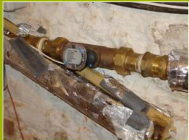
6. 'After' photo shows correct meter orientation
