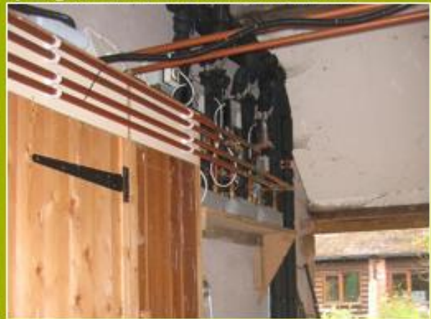
4. The pipework was wrongly declared as internal. It is external pipework as it is in an open corridor.
