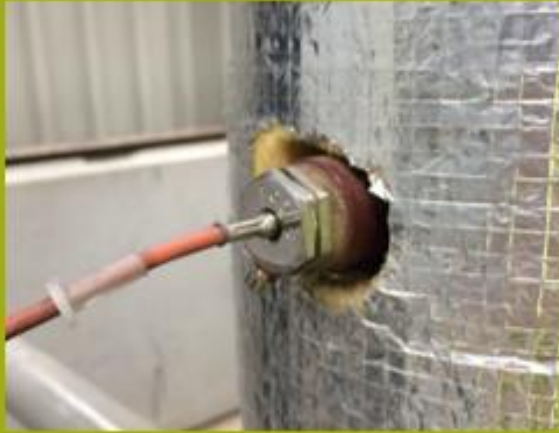
1. The sensor is installed incorrectly. Also a security tag should be attached
