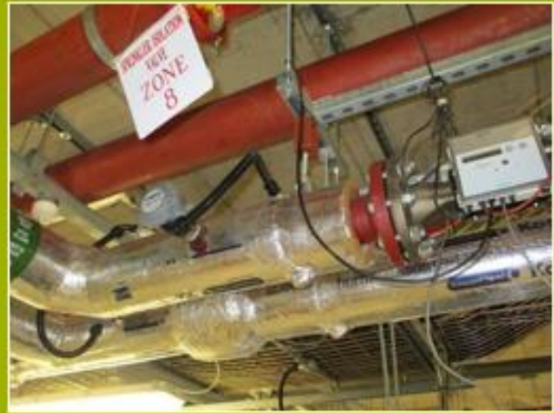
2. The meter is in the flow pipe rather than the return pipe. The flow pipe is clearly identified as seen by the green label and the witness mark arrow.
