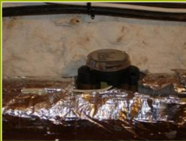
5. 'Before' photo shows incorrect meter orientation
