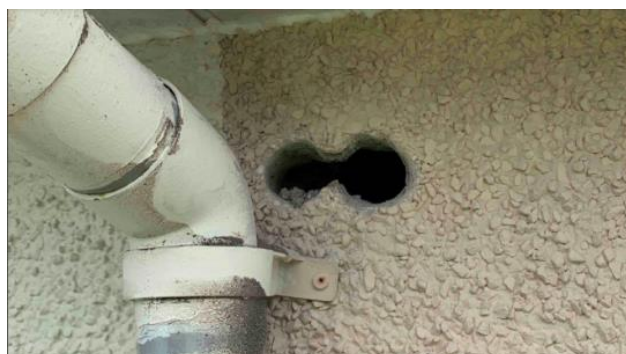
Figure 4 - Evidence of drill holes used for installation of cavity brush
