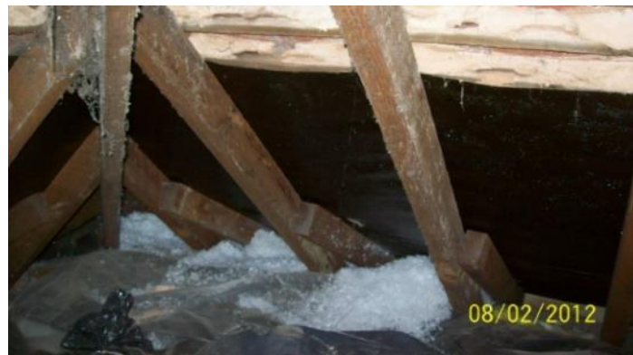
Figure 5 – Evidence of insulation material visible from the loft space
