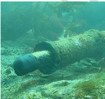
Figure 6: Capped Subsea Cable
