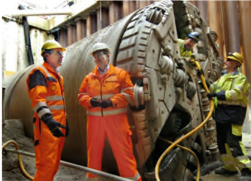
Figure 12: Successful breakthrough of the Herrenknecht SPB into a shallow piled reception pit – Corrib, Ireland
