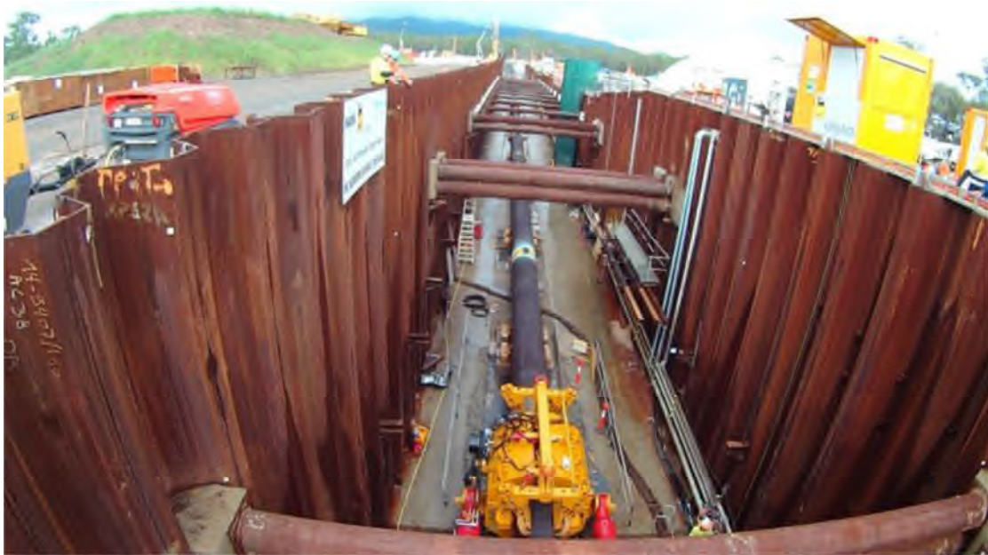
Figure 14: Pipeline threading using long pipe strings and Herrenknecht Thruster Rig – Curtis Island, Australia
