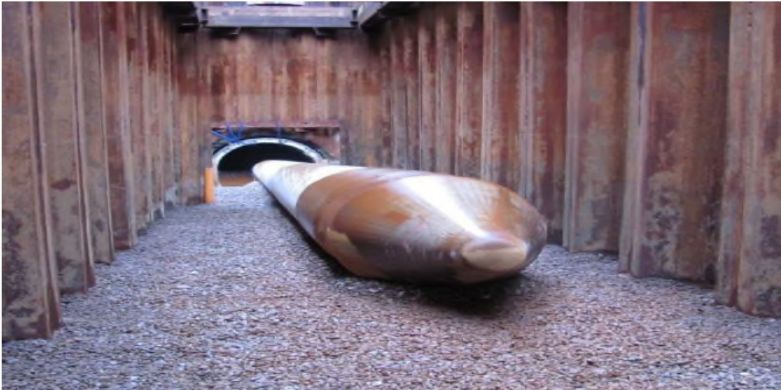
Figure 13: The 48” gas pipe emerging at reception – Ems tunnel
