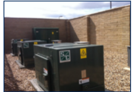
SSET1008 3 x 25kW/25kWh Lithium ion batteries
