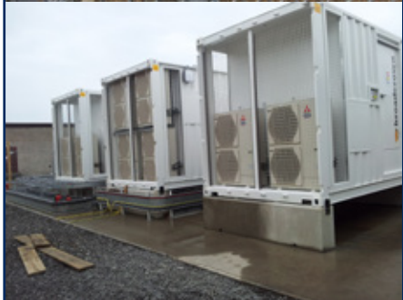
SSET1007 2MW/500kWh Lithium ion battery
