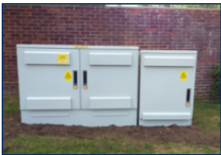
NTVV 25 x 36kW/12.5kWh Lithium ion batteries
