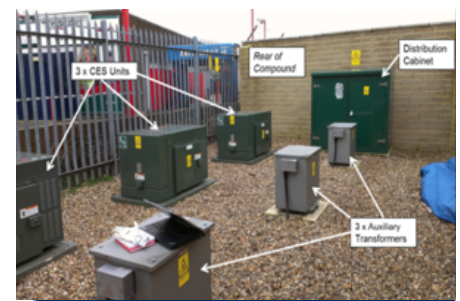
Figure 14 Finished site – 3 CES units and auxiliary transformers
