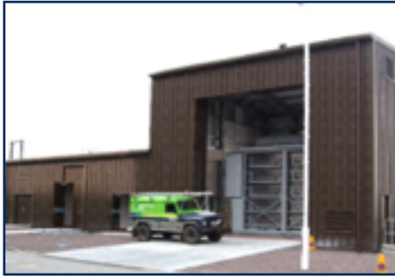
SSET1001 1MW/6MWh Sodium Sulphur battery
