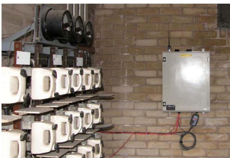
Figure 5. Enhanced secondary substation monitoring device installed in SPEN
