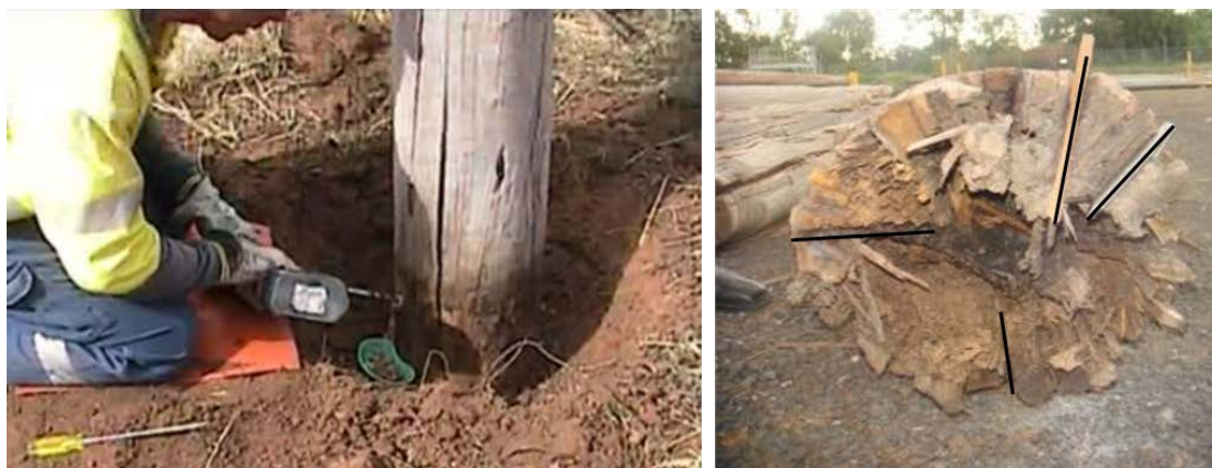
Figure 16 - Invasive Pole Strength Test and Resulting Pole Damage
