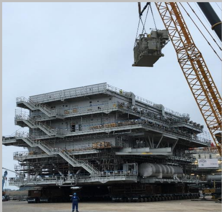
Offshore Substation Topside
