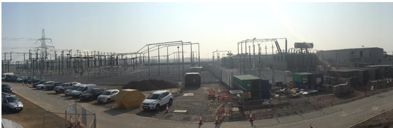
Necton substation; where the power from the wind farm is exported into the National Grid overhead lines
