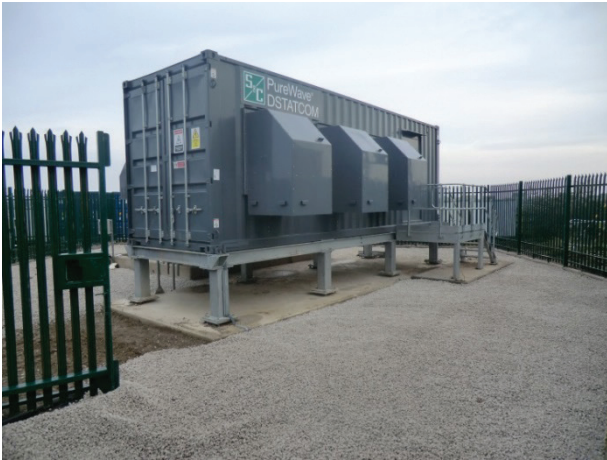
Figure 20 – DStatcom at Trusthorpe primary substation – Photo
