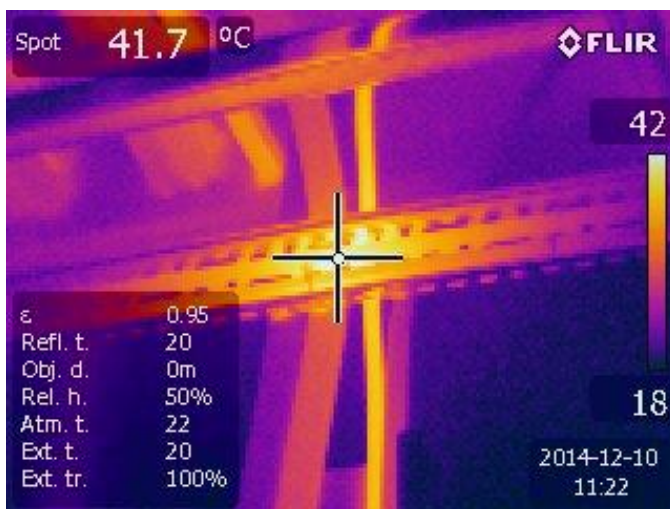
Figure 4: Picture showing temperature differential caused by induction heating in a cable support
