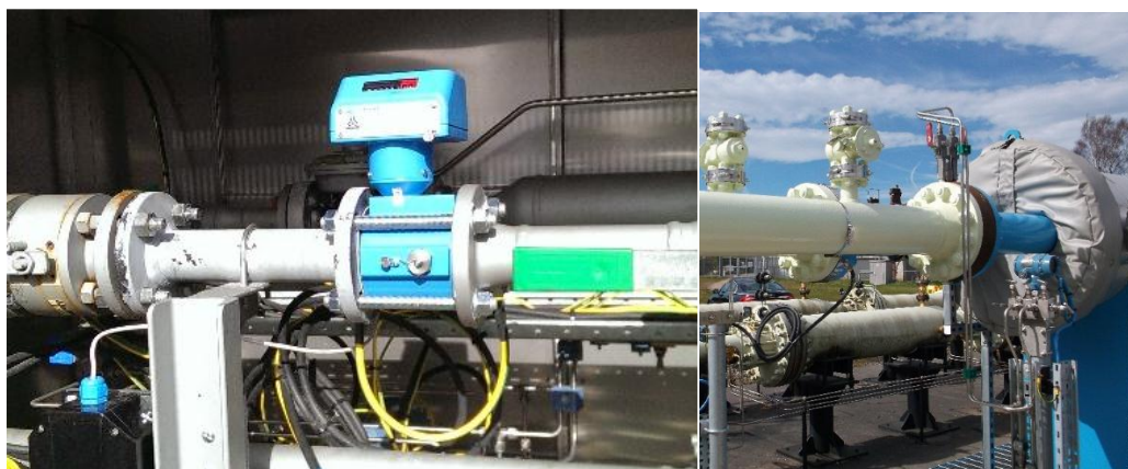
Figure 11. Example of gas meter monitoring and site inlet temperature monitoring
