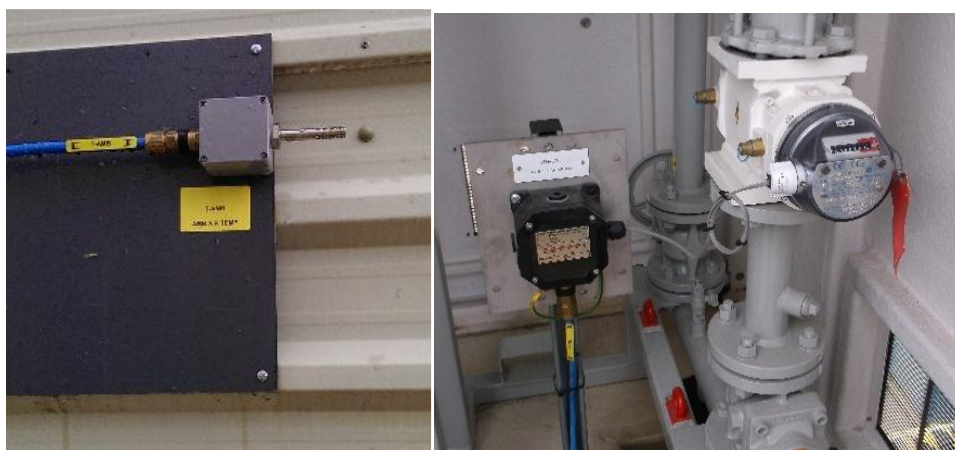
Figure 12. Examples of outdoor air temperature sensor and gas meter monitoring
