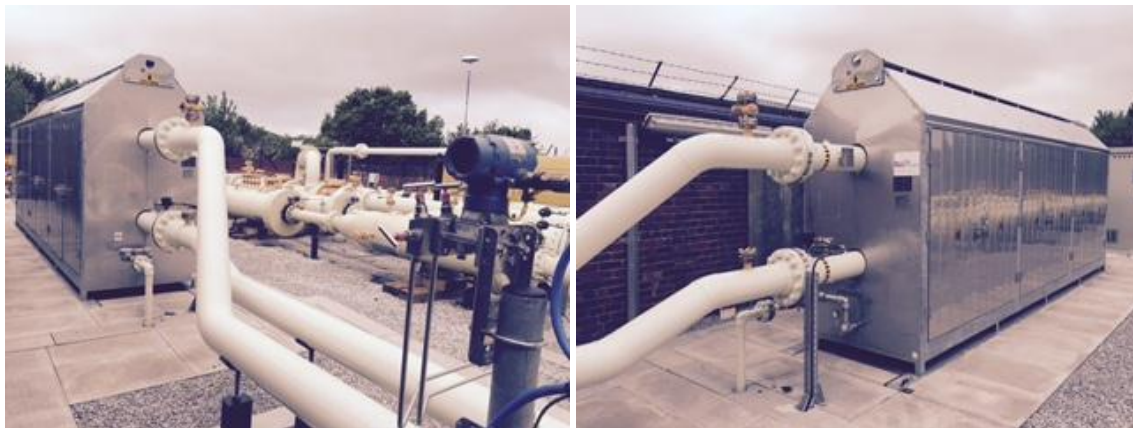
Figure 3. Small Hotcat installed at Crossgates.
