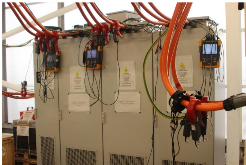
Figure 2. Picture of Prototype Multi-Terminal PED wired up for Testing at PNDC
