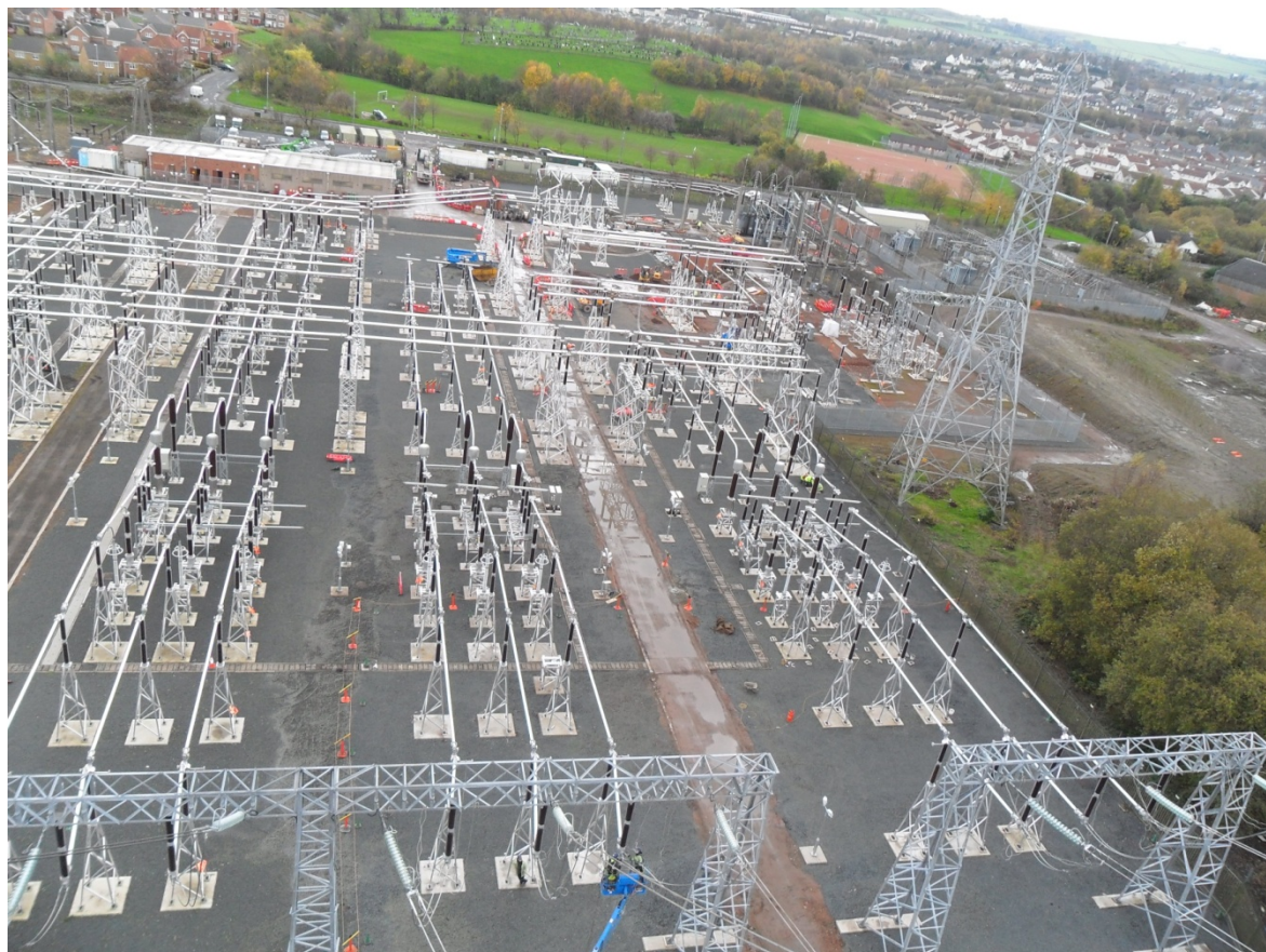
Figure 4.4 – View of 275kV Switchgear Bays (Longannet then Easterhouse from left)
