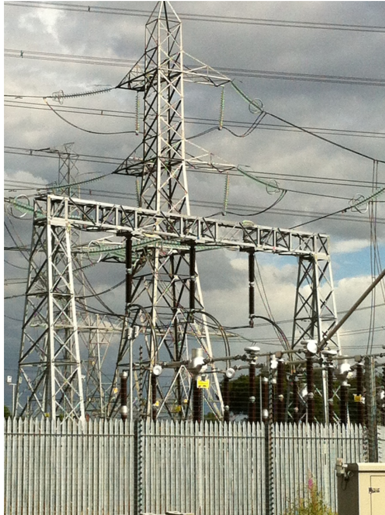
Figure 4.8 – Longannet Circuit Line Gantry
