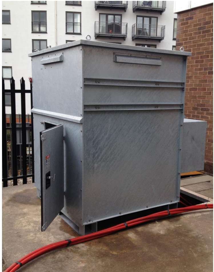
Figure 5-9: Resistor on site
