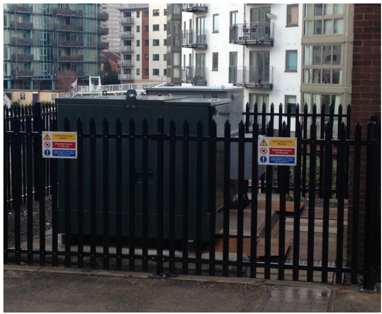
Figure 5-10: AFLM Installation at Ladywood – Side View
