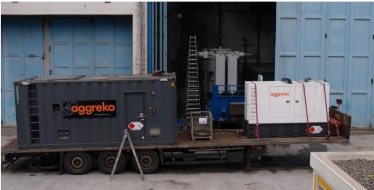
Figure 9 FCL and Generator in Short Circuit Test Laboratory
