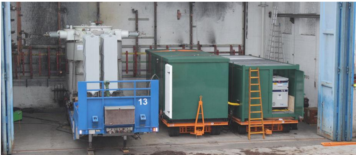
Figure 7 The FCL (left) and Auxiliary Enclosures (right) in the Short Circuit Test Cell
