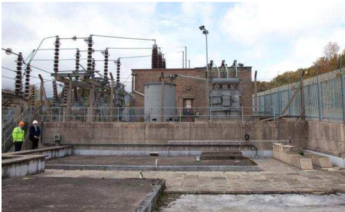
Spare supergrid transformer bay. The SFCL is to be mounted on the far plinth.
