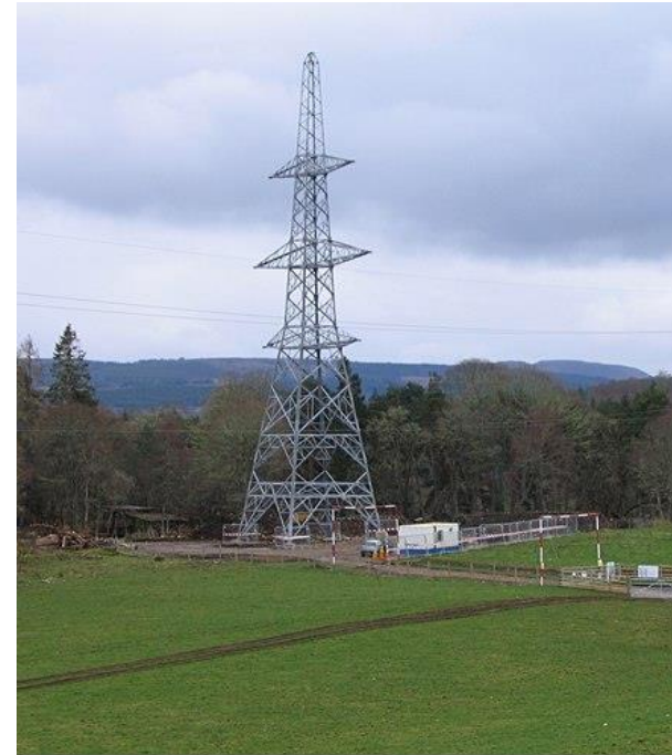
First new pylon completed on the Beaully-Denny power line © Copyright Craig Wallace and licensed for reuse under this Creative Commons Licence .
