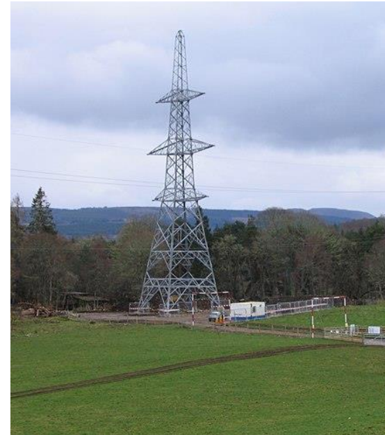
First new pylon completed on the Beauly-Denny power line © Copyright Craig Wallace and licensed for reuse under this Creative Commons Licence .
