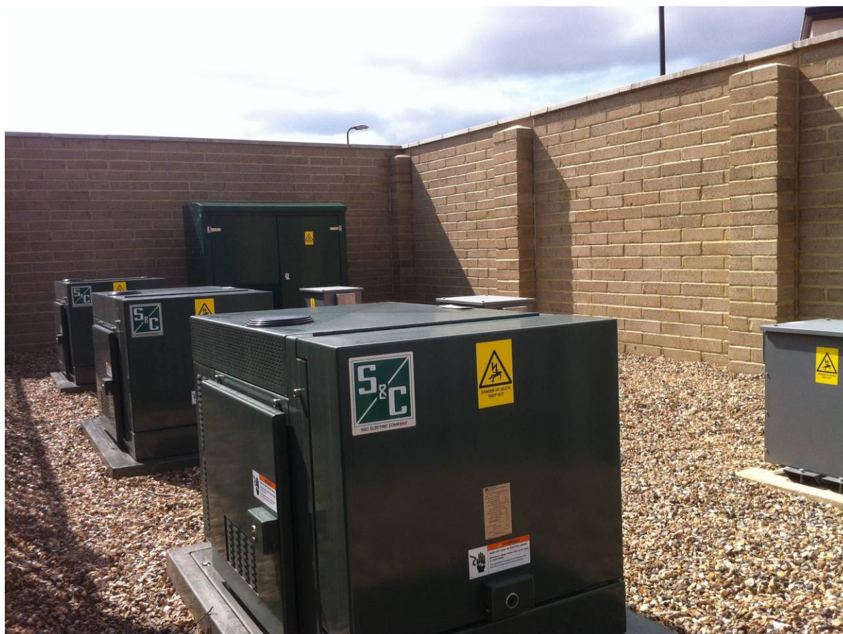
Figure 1 – Close up view of CES units in compound – showing the 3 above ground PCS units in the foreground and LV cabinet in background
