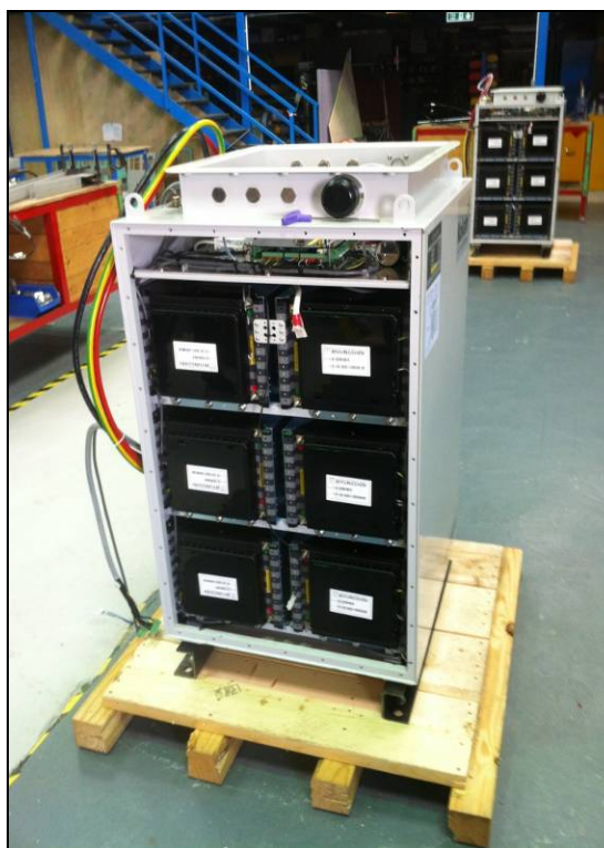
Figure 3: Battery module with side panels removed at S&C factory, Swansea
