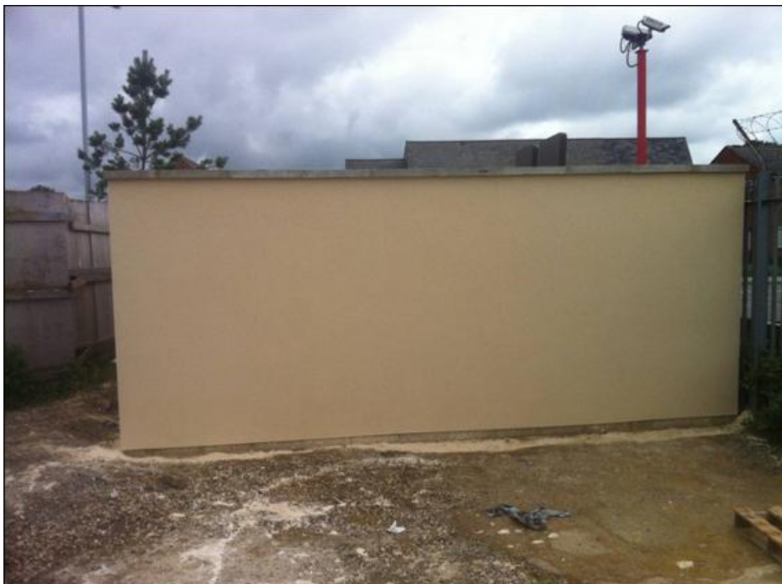
Figure 14 - External view of rendered perimeter wall (rendered to blend-in with the nearby Zero Carbon Homes using the same colour and style)
