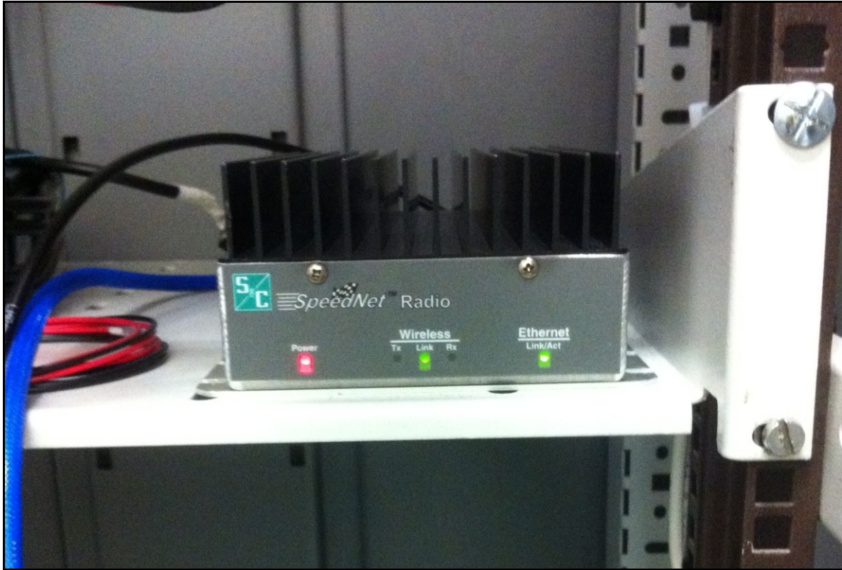
Figure 20: View of SpeedNet Radio in Chalvey RTS Room
