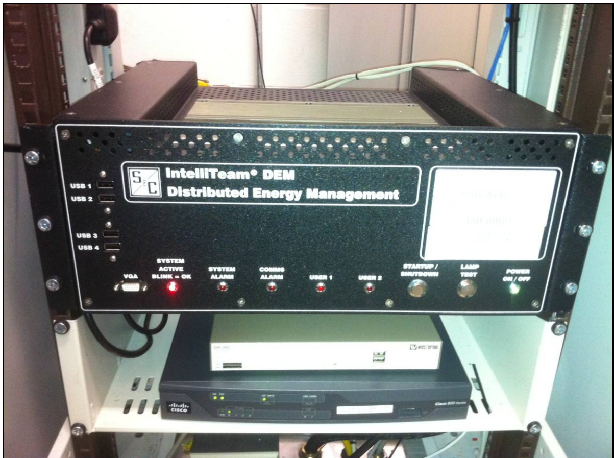
Figure 18 - DEM plus Cisco router for remote access installed at Chalvey 11kV substation
