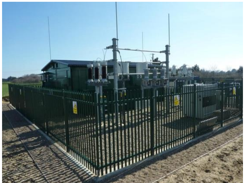
Figure 1 the energy storage installation as built
