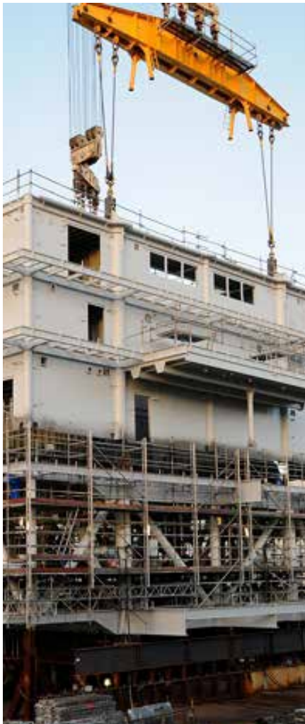
- Westermost Rough offshore platform. Image: DONG Energy
