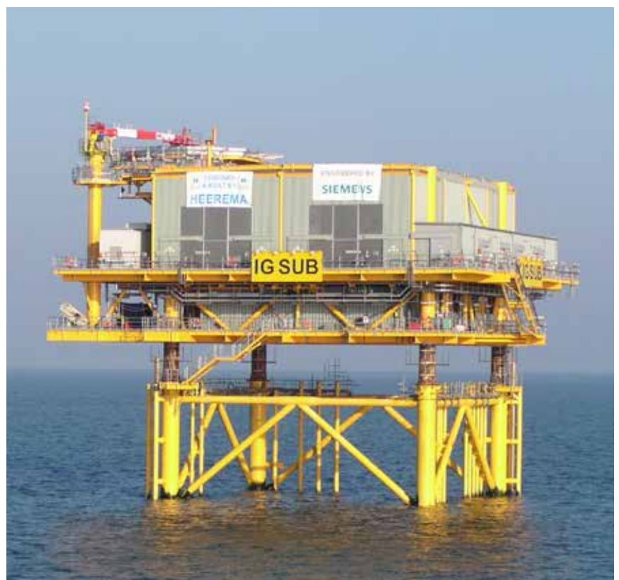
- Greater Gabbard offshore substation. Image: Greater Gabbard Offshore Winds Limited
