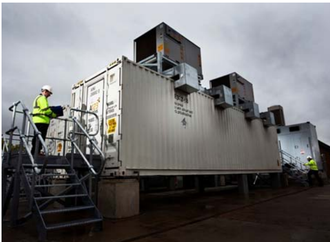
Figure 1 - Rise Carr 2.5MVA battery and inverters
