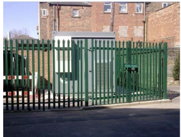
Figure 2 - High Northgate 100 kVA battery
