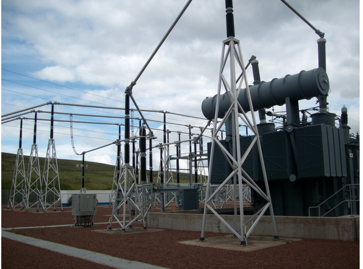
Figure 4.29 – SGT1B 400/26.5kV Transformer
