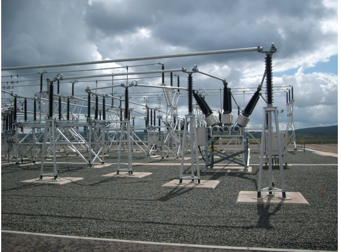
Figure 4.16 –132kV Bus Coupler Bay
