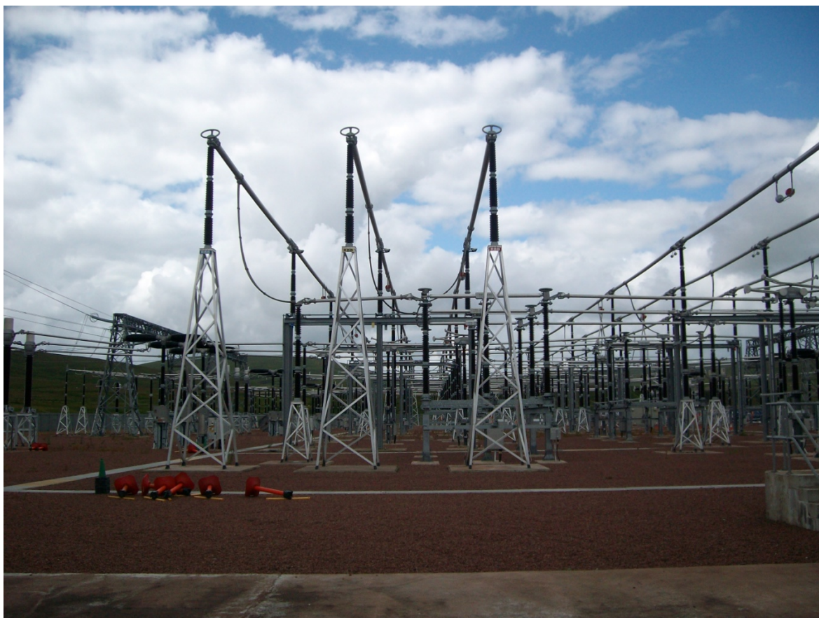
Figure 4.25 – View of 400kV Switchyard (main & reserve busbars)
