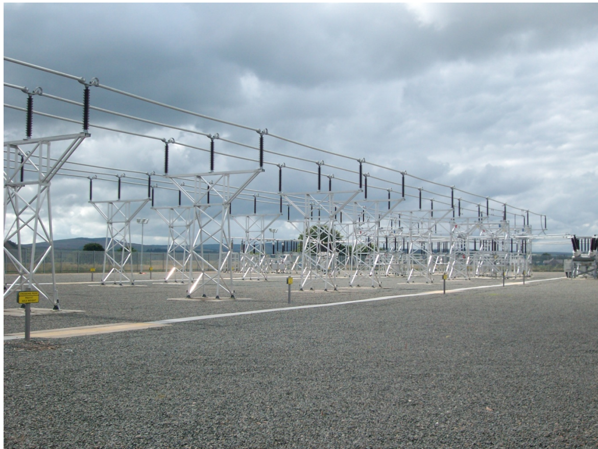
Figure 4.11 – View of 132kV Switchyard (main & reserve busbars)
