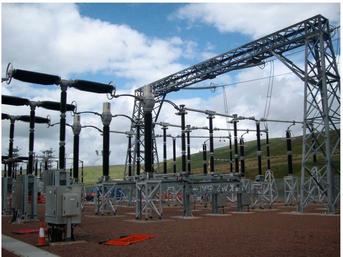
Figure 4.27 – Incoming Coalburn Line Termination
