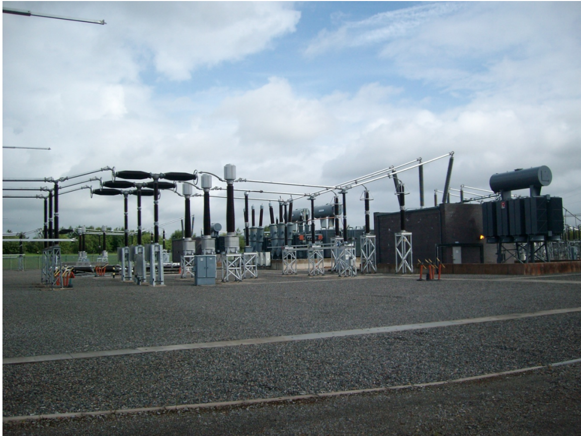
Figure 4.36 – SGT2 400/132kV Transformer
