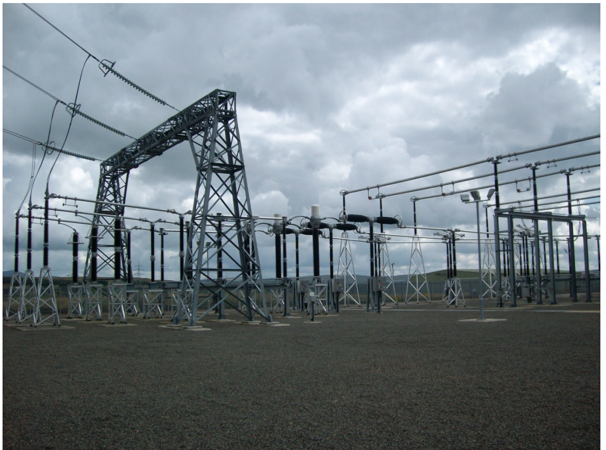
Figure 4.13 – Incoming 400kV Elvanfoot Line Termination
