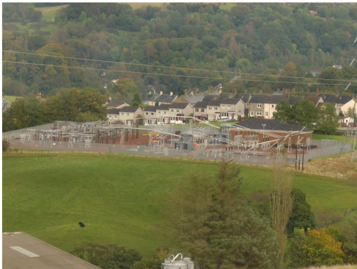
Figure 4.20 – View of Linmill Substation
