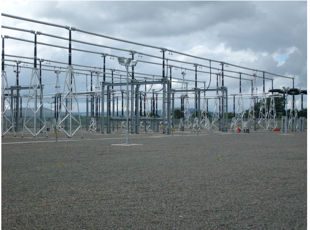
Figure 4.10 – View of 400kV Switchyard (main & reserve busbars)
