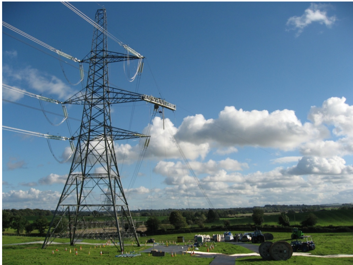
Figure 4.38 – Re-conductoring of 400kV Eccles – Stella West Overhead Line Circuits
