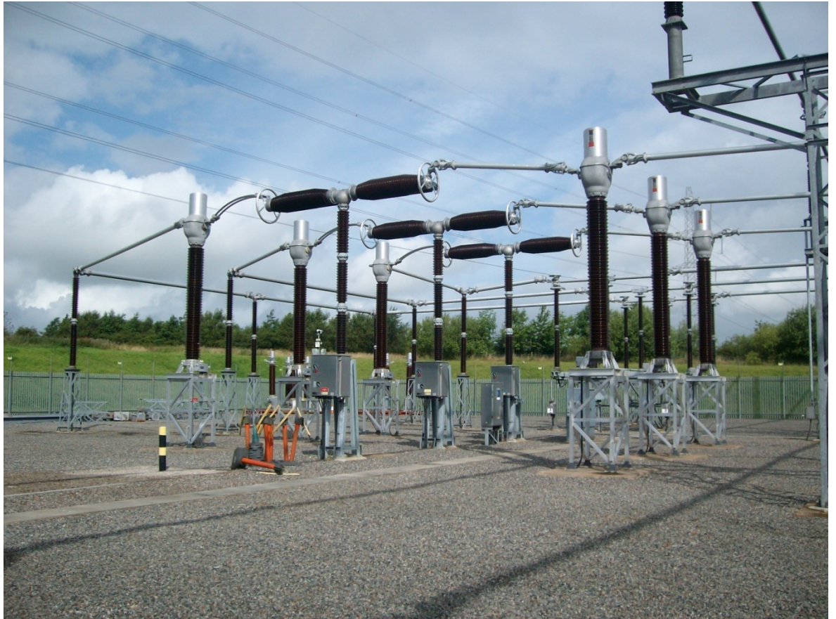
Figure 4.35 – 400kV Bus Coupler Circuit Breaker & CT's
