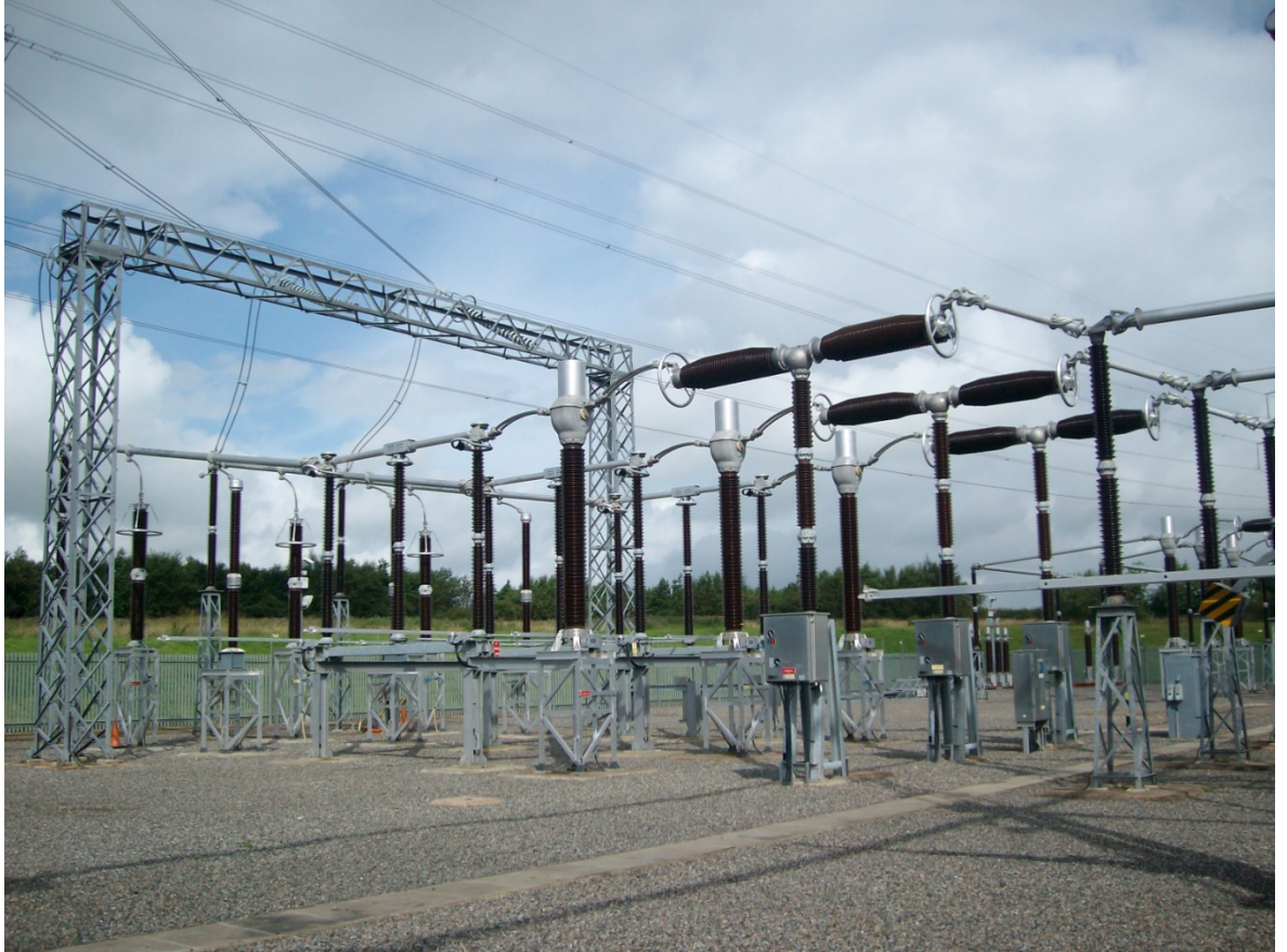
Figure 4.34 – Incoming 400kV Elvanfoot Line Termination
