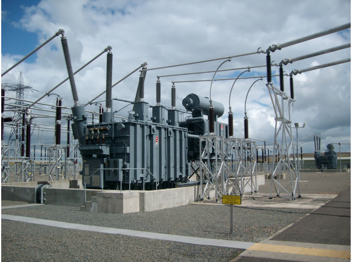
Figure 4.15 – SGT1 400/132kV Transformer
