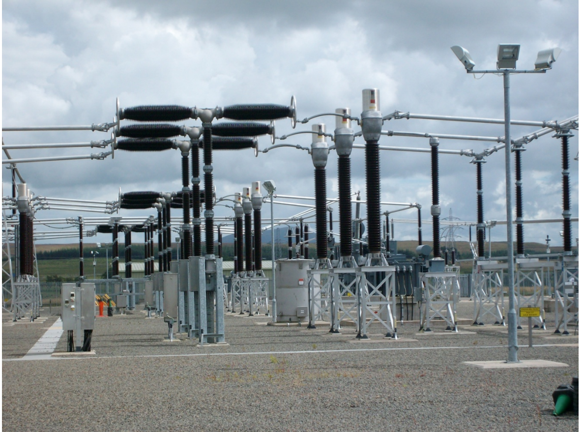
Figure 4.14 – 400kV Circuit Breaker & CT's
