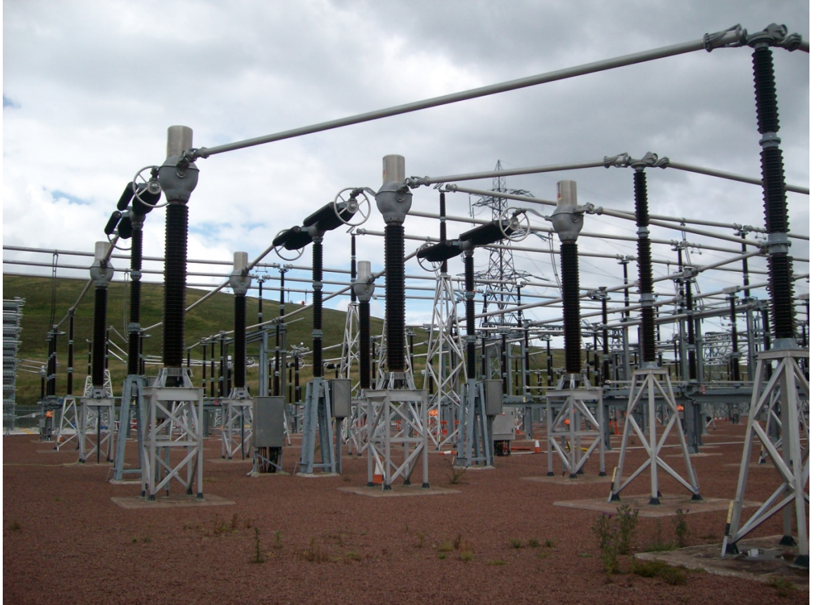
Figure 4.28 – 400kV Bus Coupler Circuit Breaker & CT's
