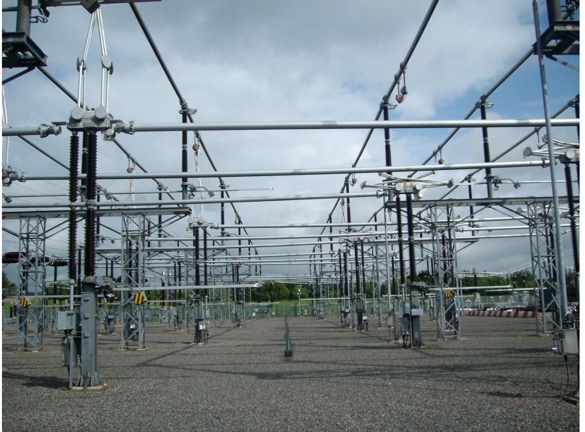
Figure 4.33 – View of 400kV Switchyard (main & reserve busbars)
