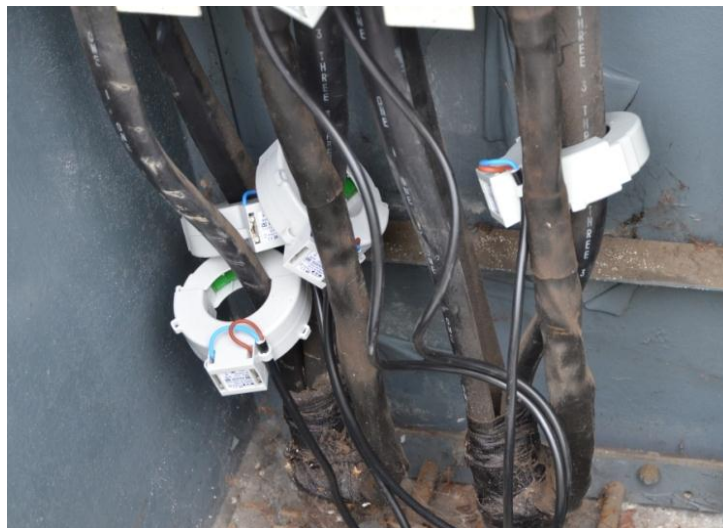
Figure 12: PowerSense split core CTs around LV phase cores (WPD).
