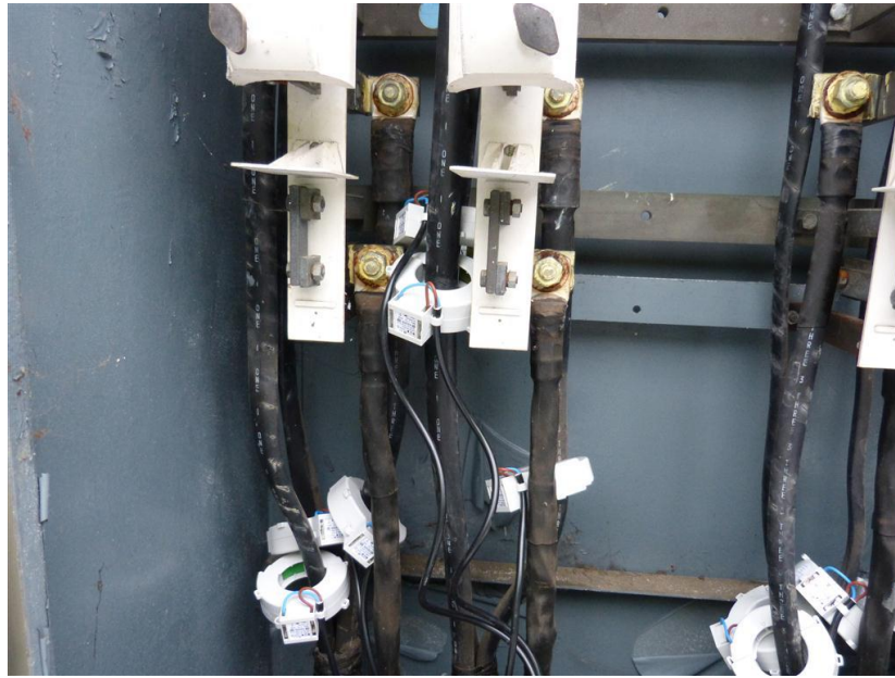
Figures 14: Example of CT installation high up cables due to spacing restrictions. (WPD)
