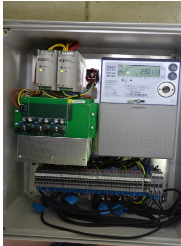
Figure 22: Data aggregation electronic boards and EDM I Atlas Mk10A meter inside the Haysys metrology unit.
