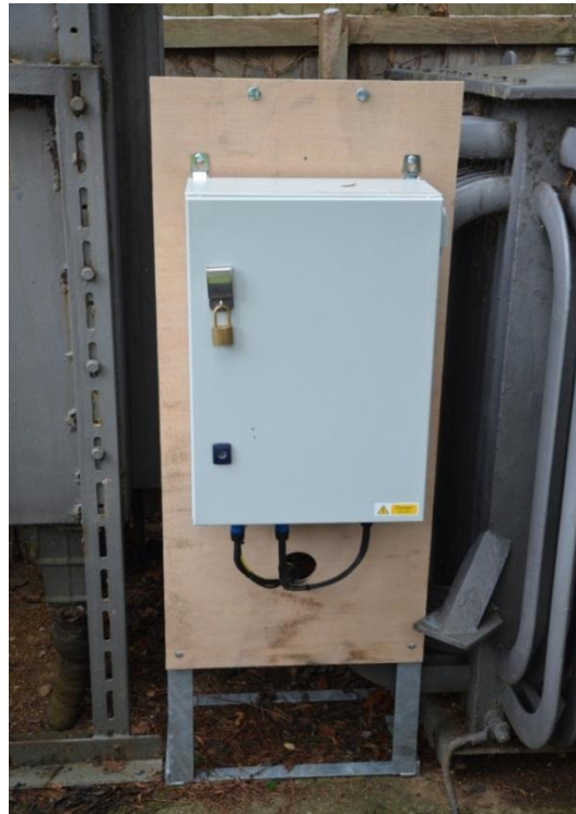
Figure 2: GMC i-Prosys metrology unit installed in outdoor substation. (WPD)
