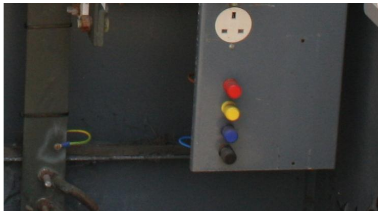
Figure 7: LV Cabinet with 3 phase test point
