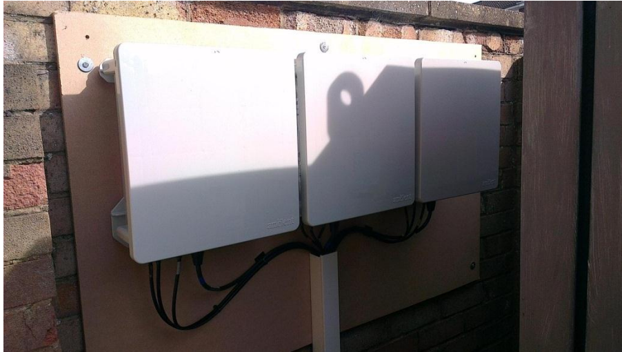
Figure 20: Ambient metrology units, one for each LV way. (WPD)
