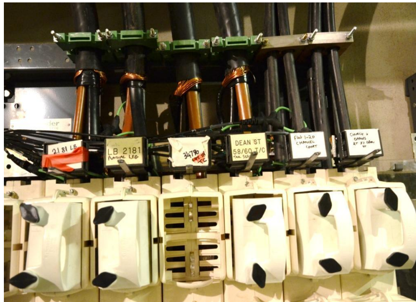
Figure 3: GMC i-Proslys Rogowski coils installed around tightly spaced cable cores.
