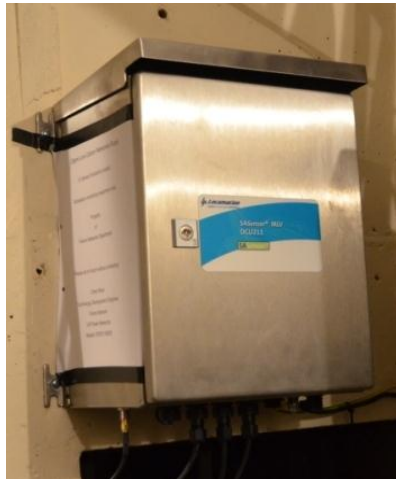
Figure 26: Locamation metrology unit. (UKPN)
