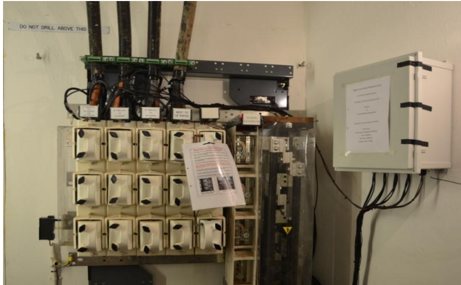
Figure 24: Haysys monitoring solution installed in substation. (UKPN)
