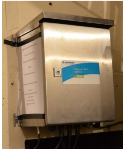
Figure 26: Locamation metrology unit. (UKPN)
