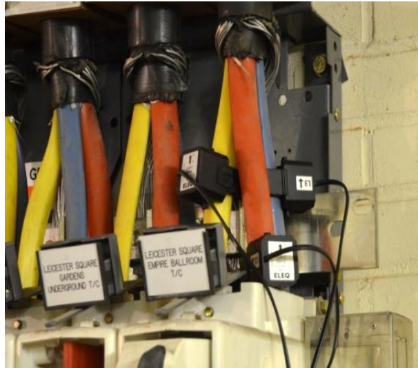
Figure 27: Locamation split core CTs around individual phase cores. (UKPN)
