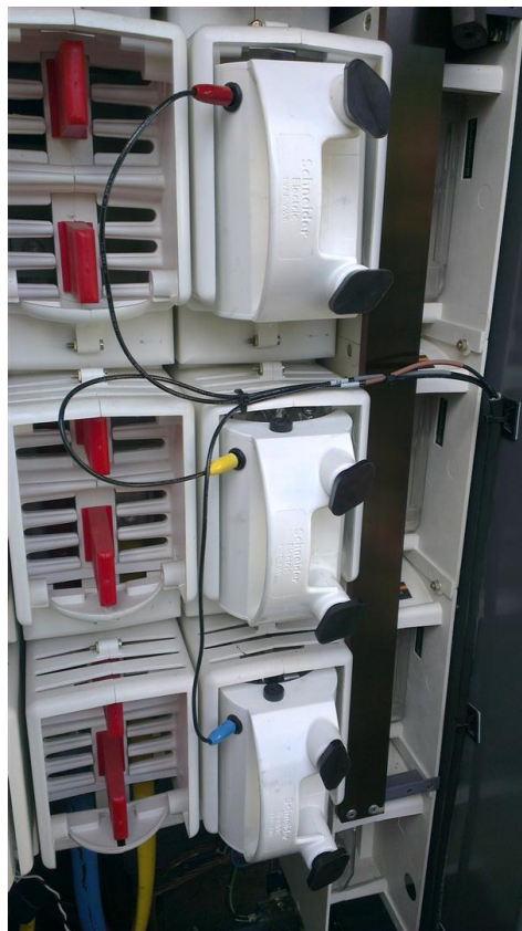
Figure 11: Modified fuse carrier handles installed on spare leg in pillar
