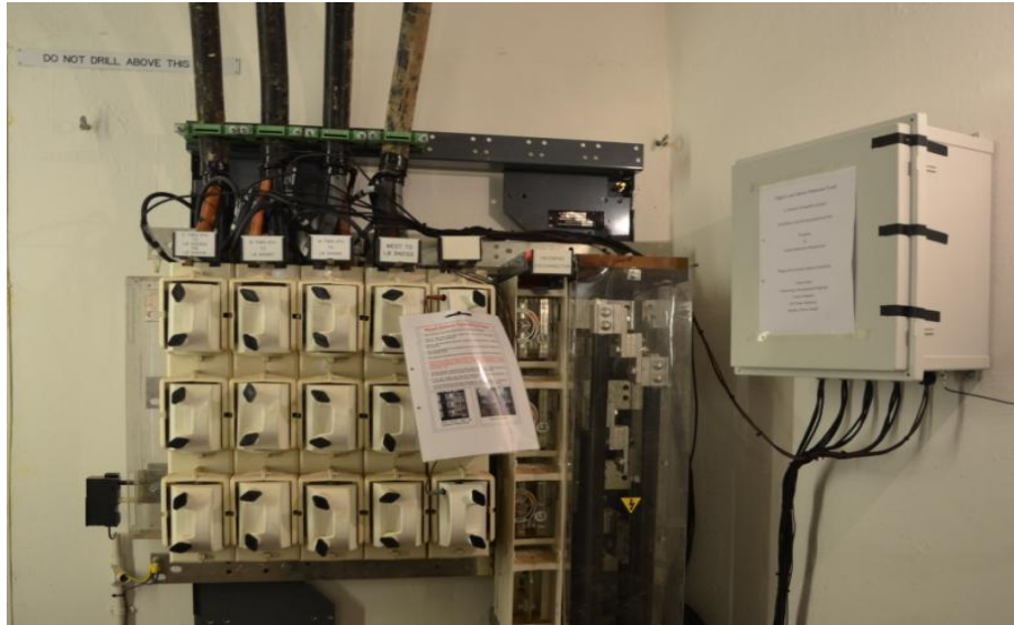
Figure 24: Haysys monitoring solution installed in substation. (UKPN)
