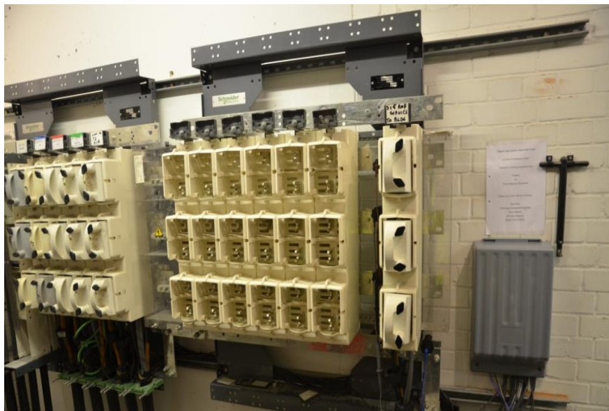
Figure 6: The GridKey MCU with the sensors and voltage leads connected. (UKPN)
