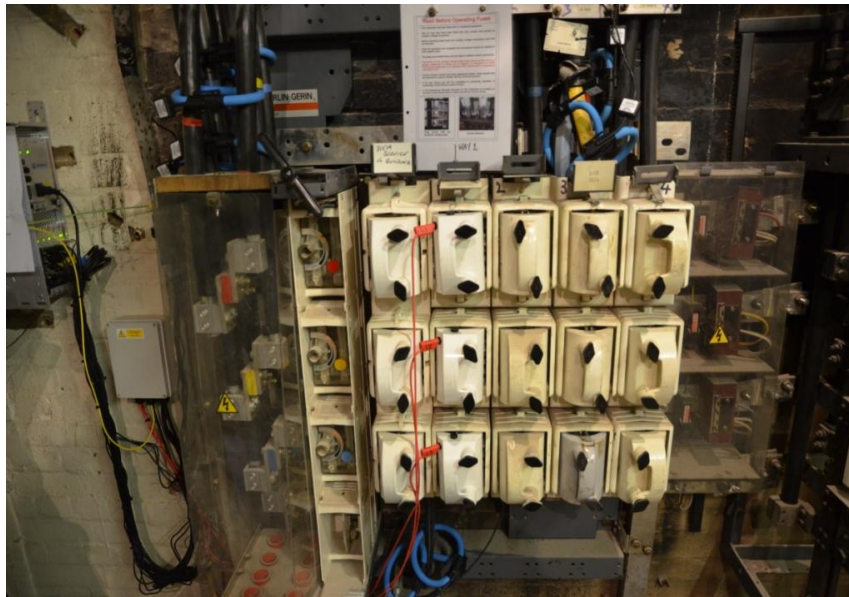
Figure 11: Current monitoring solution installed in UKPN substation.
