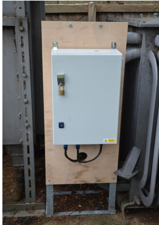
Figure 2: GMC i-Prosyst metrology unit installed in outdoor substation. (WPD)
