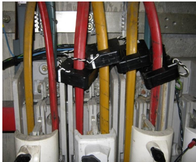
Figure 19: Ambient CTs around core conductors on an open LV board. (UKPN)
