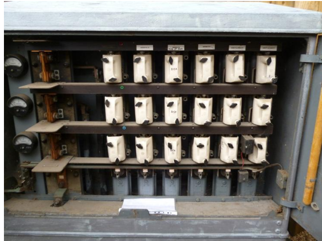
Figure 4: LV cast iron cabinet with compound filled tiered cable terminations.
