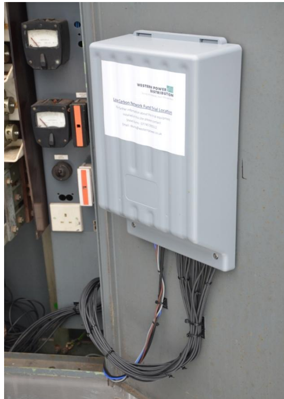
Figure 5: Sensor cables and voltage/power cables coming into the metrology unit (WPD).
