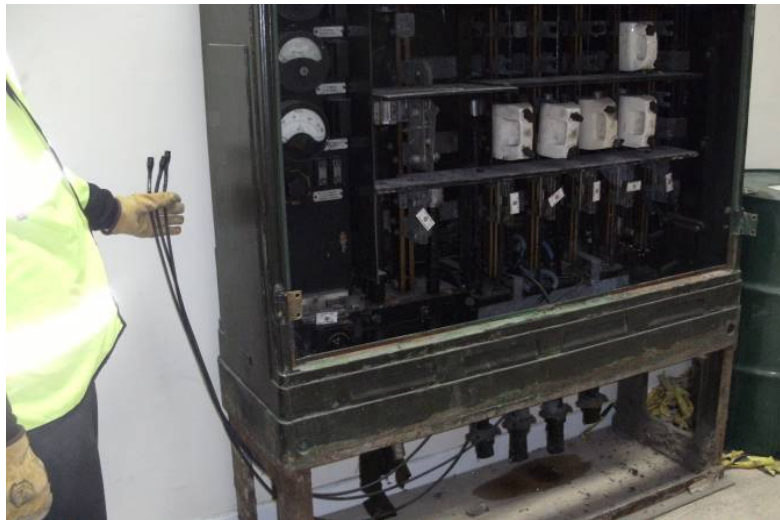
Figure 4 Traditional open LV pillar
