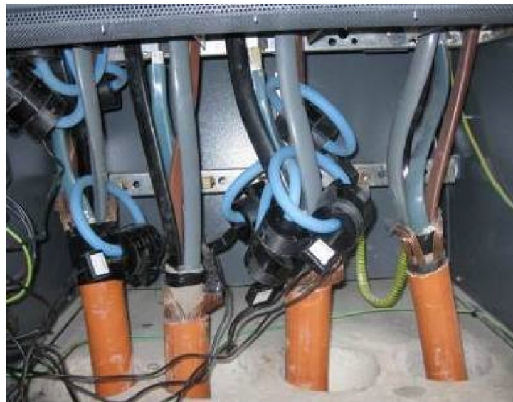
Figure 5 CURRENT Group Rogowski Coils (blue) 'live installed' at two LV feeders
