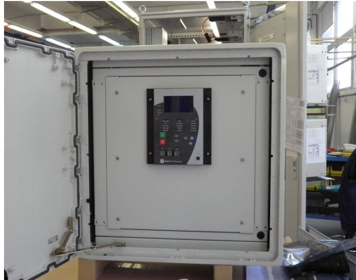
Figure 10 GE C650 Relay Installed in Protective Cabinet
