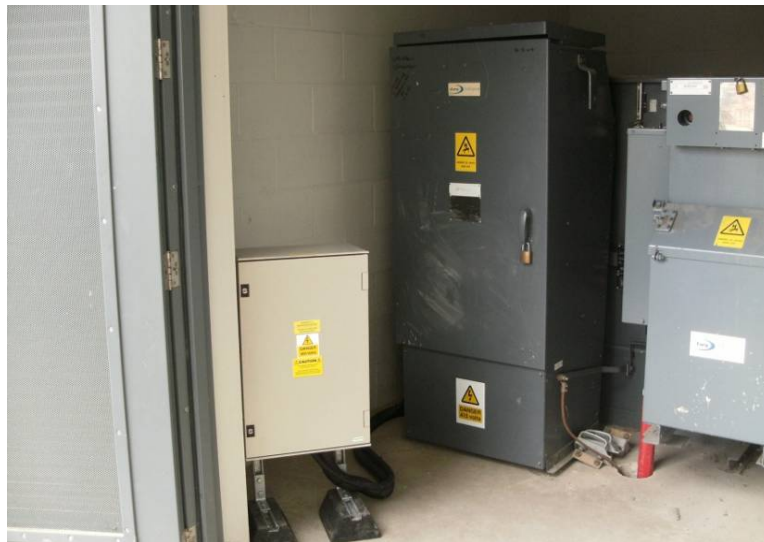
Figure 7 CURRENT Group equipment (unit at left of picture) as installed at Chalvey S/S
