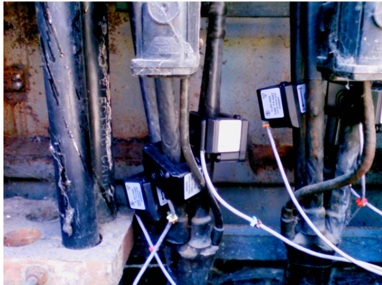
Figure 2 GridKey CURRENT transducers installed on LV feeder cables
