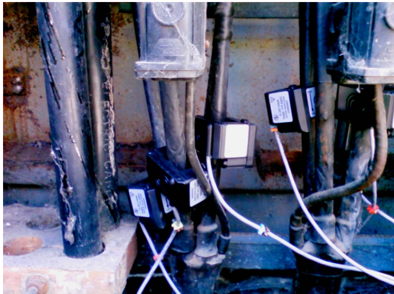
Figure 13 GridKey current transducers installed on LV feeder cables
