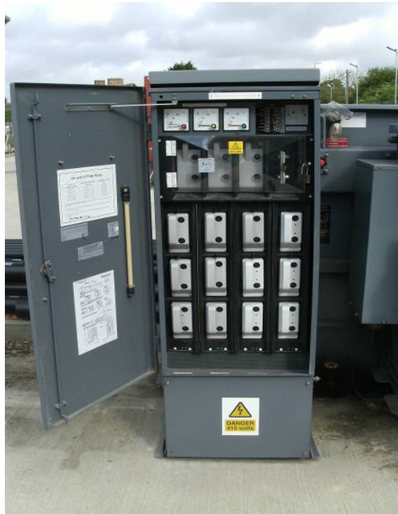
Figure 3 Modern shrouded/screened type LV cabinets
