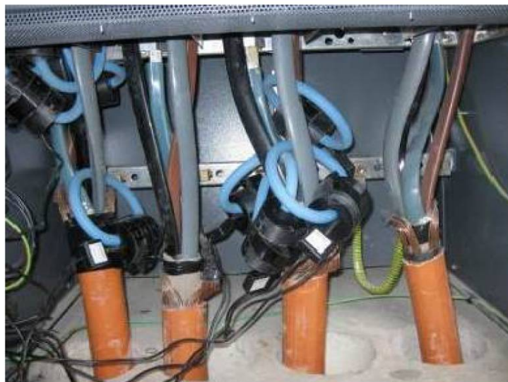
Figure 1 CURRENT Group Rogowski Coils (blue) 'live installed' at two LV feeders
