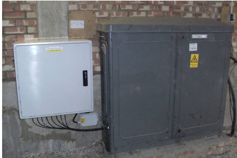
Figure 12 GE Cabinet Mounted at Service Yard D Substation
