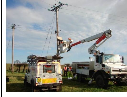
Figure 4: Overhead line rating devices
