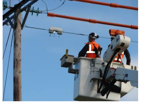
Figure 5: Overhead line rating devices
