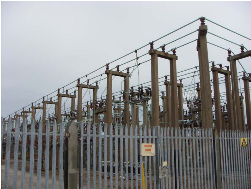
Photograph 4 – General view of the 33kV outdoor compound at Lockleaze BSP
