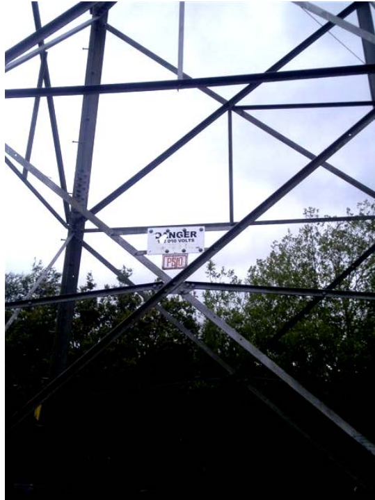
Photograph 1 – The shotgun damage to the original danger plate at tower 10
