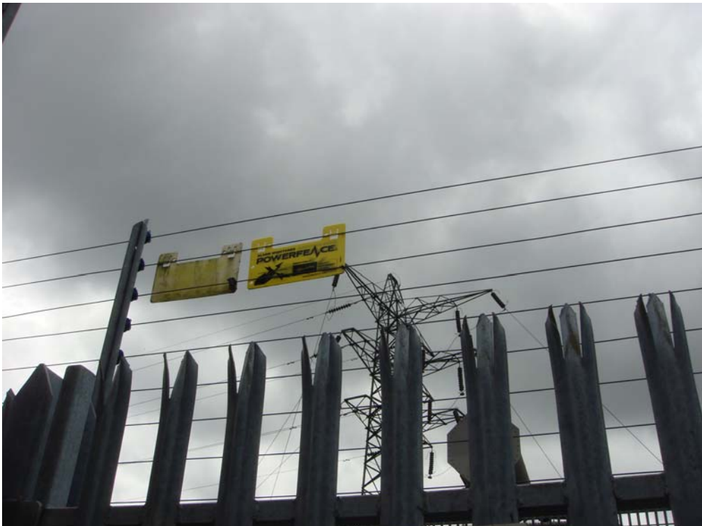
Photograph 2 – The warning signs on the electric fence
