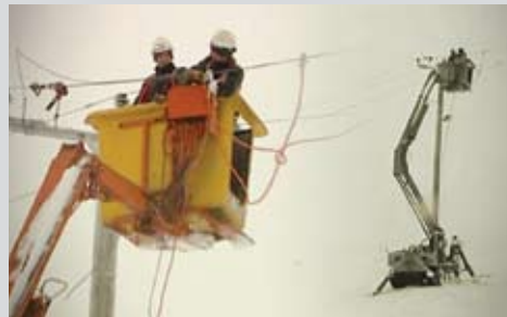
Weather damage: Wear Valley repairs
