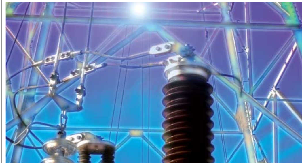
Distribution: local networks will need significant investment to be able to handle renewables growth
