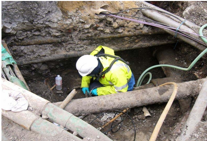
Figure 3.5 - Repair of a gas escape in the highly congested underground environment of London
