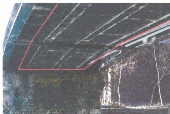
Metal casing containing six 400kV cables (within the red line), Kingsland Basin footbridge. (See also above right)
