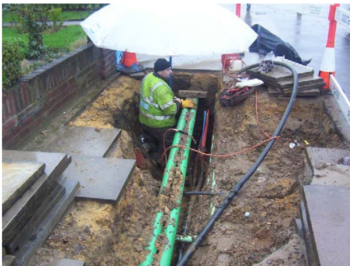
Image 4: Shows the difficulty of joining power cables underneath telecommunication cable ducts.
