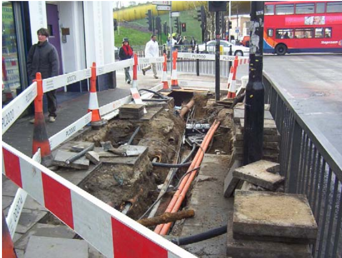
Image 5: Link box at junction showing scale of excavation, lack of immediate parking and space for spoil. Orange ducts are for highway authority traffic control equipment. Hand excavation essential to avoid damage to these.
