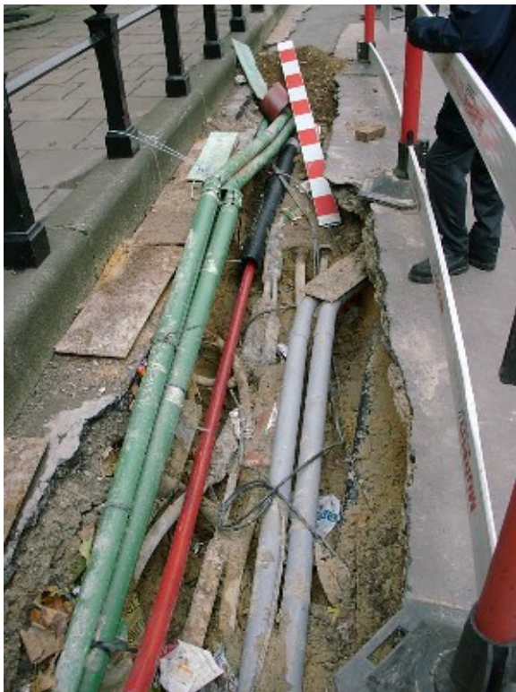
Image 6: LV cables (in centre showing joints) under/amongst telecoms infrastructure (green and grey). Hand excavation required and little space for our operatives to stand/work in.
