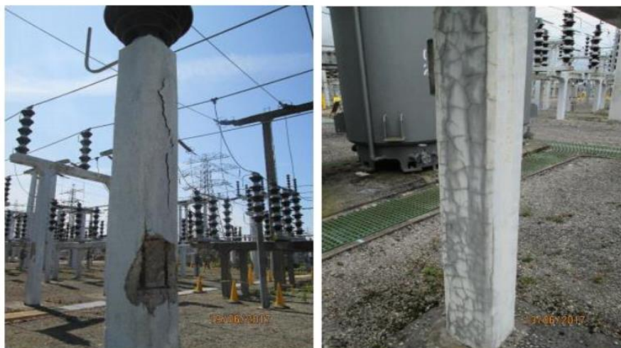
(1) 230 isolator showing typical cracking (2) 180 isolator post
