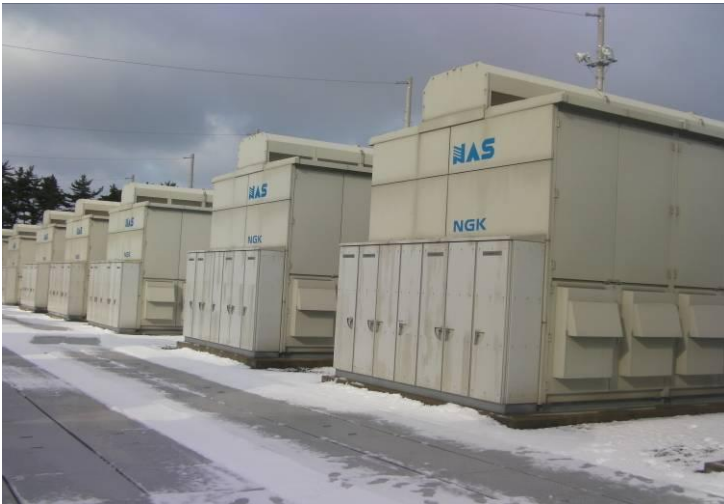
Figure 5 - 34MW battery, Rokkasho wind farm, Japan
