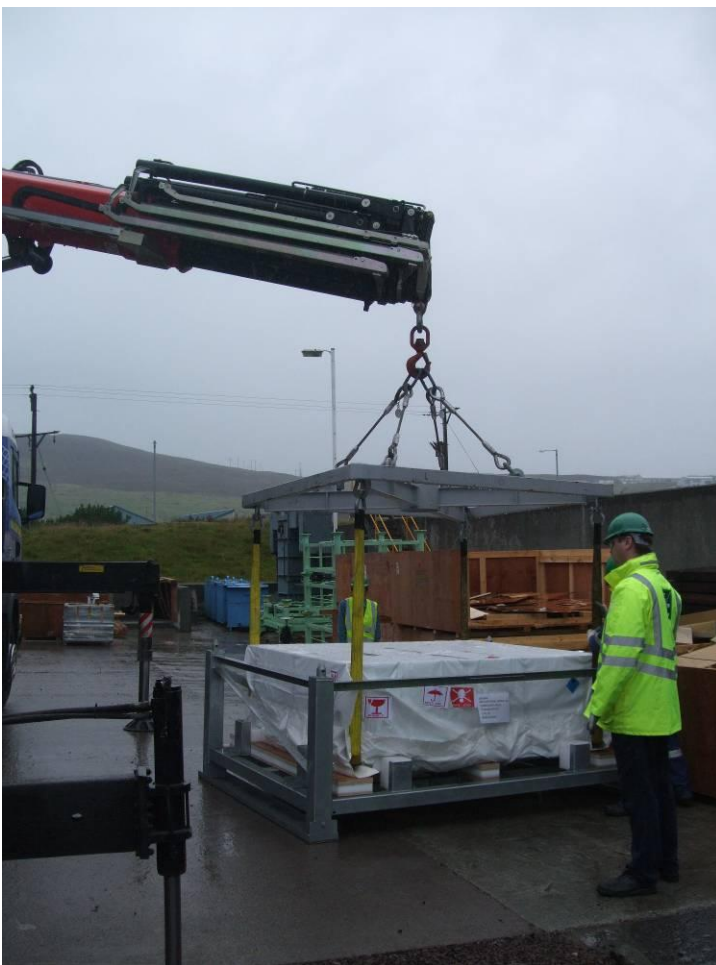
Figure 12- Battery module being removed from transportation frame
