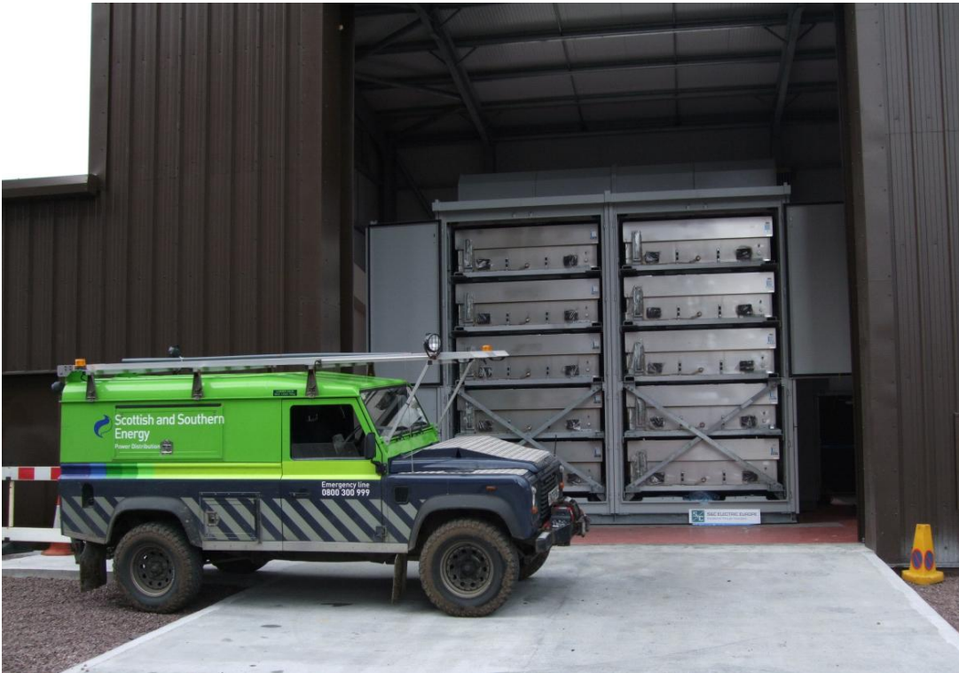
Figure 17 - NAS battery system installed at Lerwick Power Station
