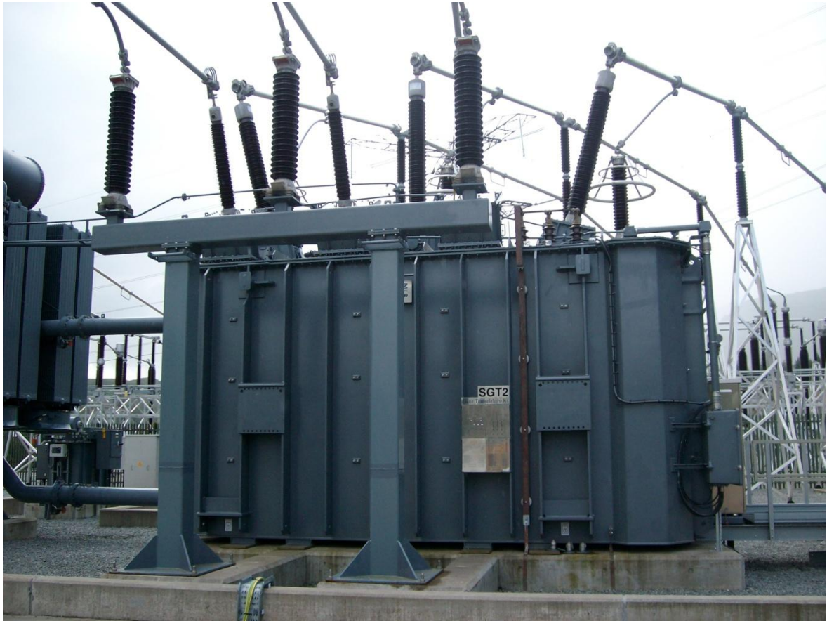
Figure 6.2 – SGT2 transformer as installed
