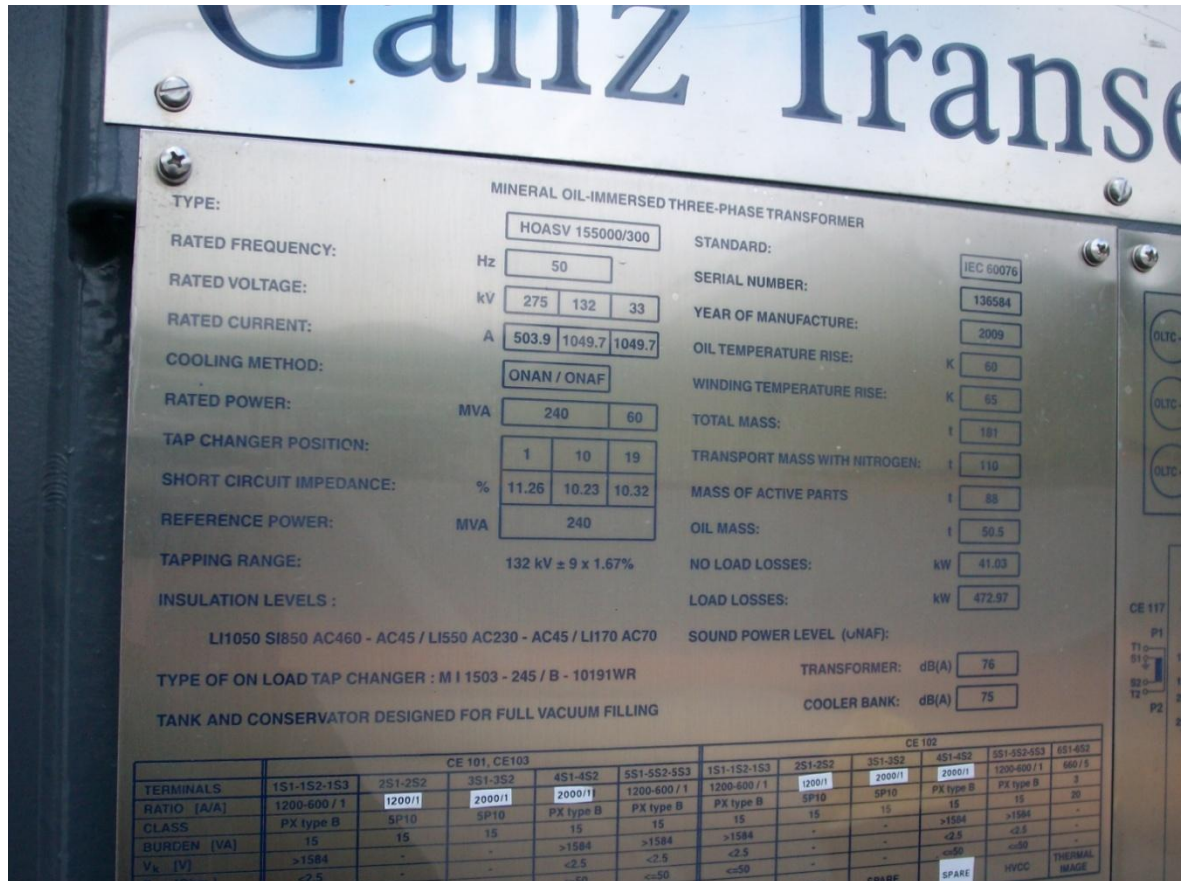
Figure 6.5 – Nameplate rating of SGT2
