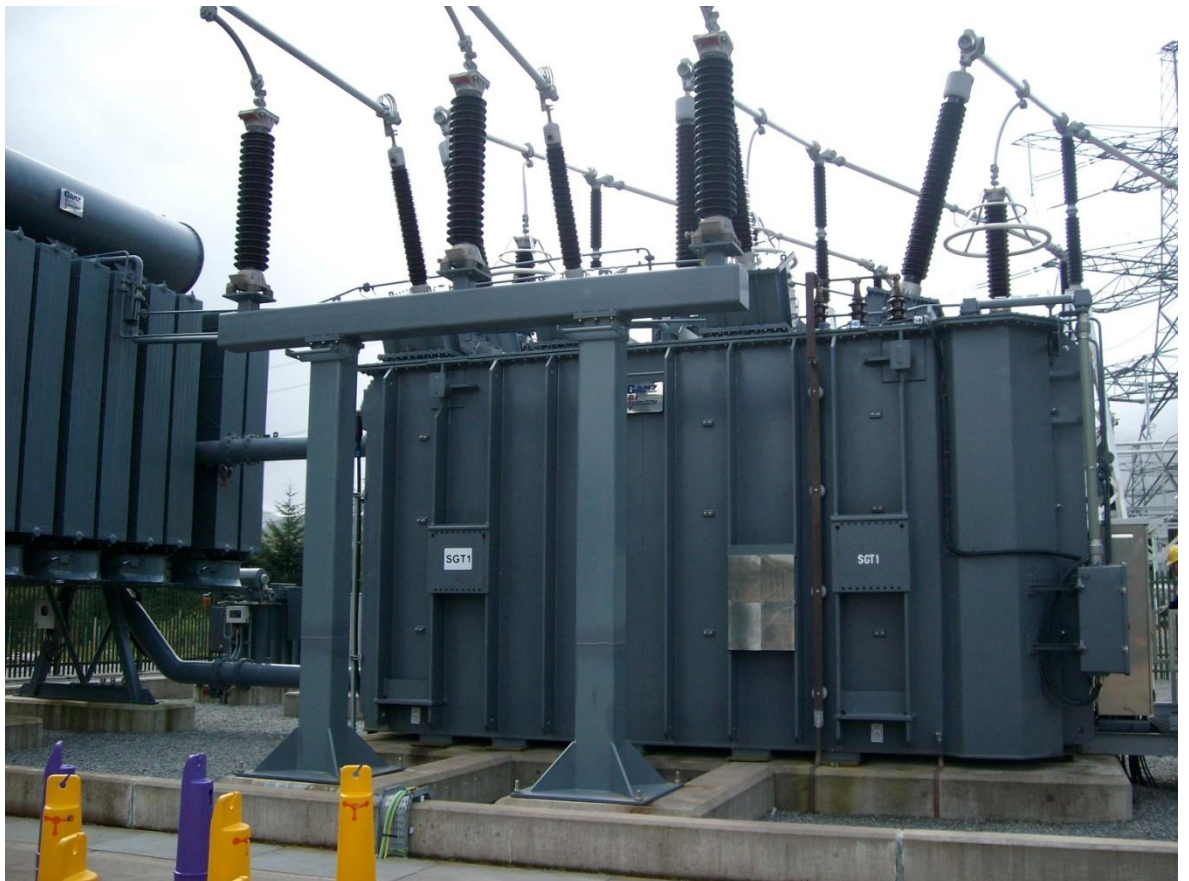
Figure 6.1 – SGT1 transformer as installed
