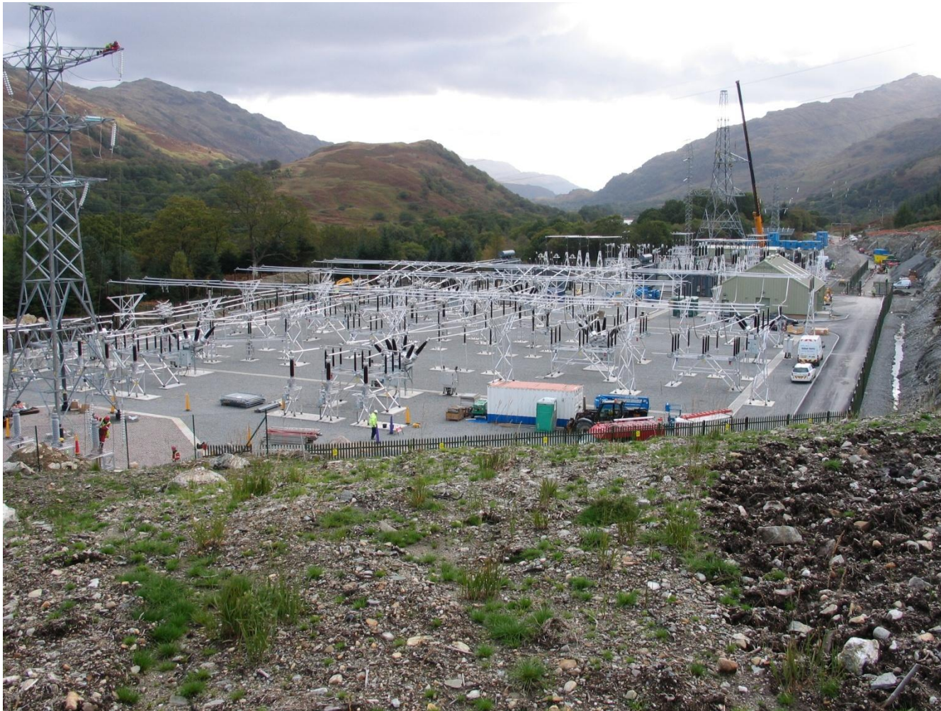
Figure 4.3 – Inverarnan Substation (near completion)
